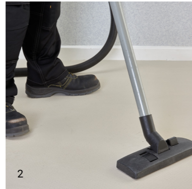
2 Sweep or vacuum the floor area, check the condition of the subfloor and make good as necessary. If the substrate is highly porous a suitable primer may be required.
